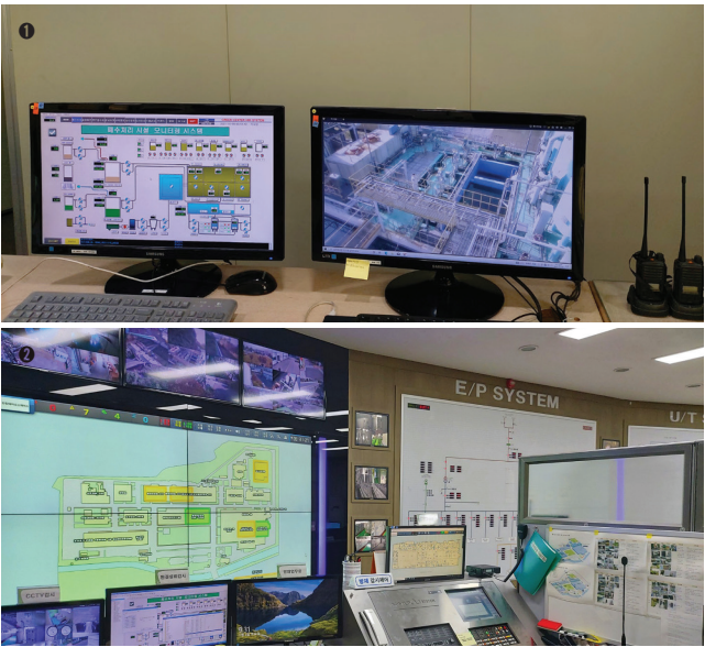
①Green Center ②Comprehensive Control Center
